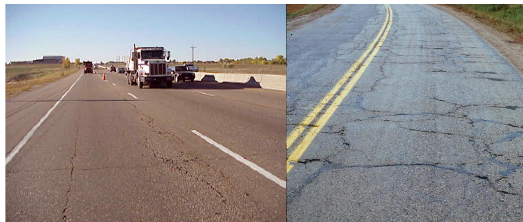
Figure 1. (a) Top-bottom cracking resulting from high axle/tire pressure on pavement surface (b) block cracking due to shrinkage of asphalt concrete from daily temperature cycling
